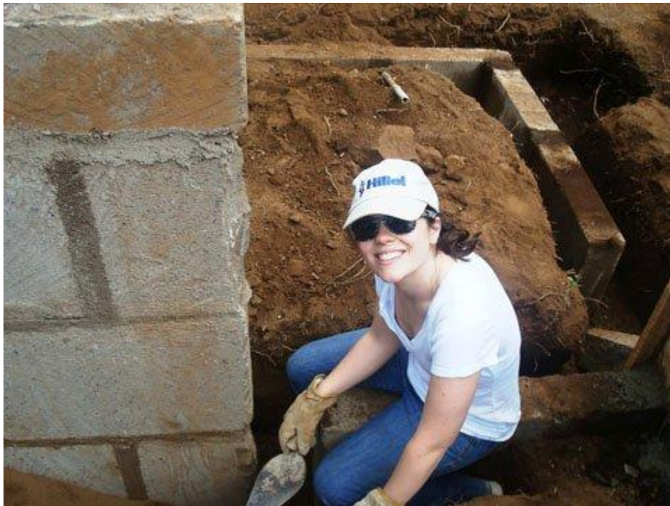
Sheila helping to build a community center during a Hillel-AJWS alternative spring break trip
